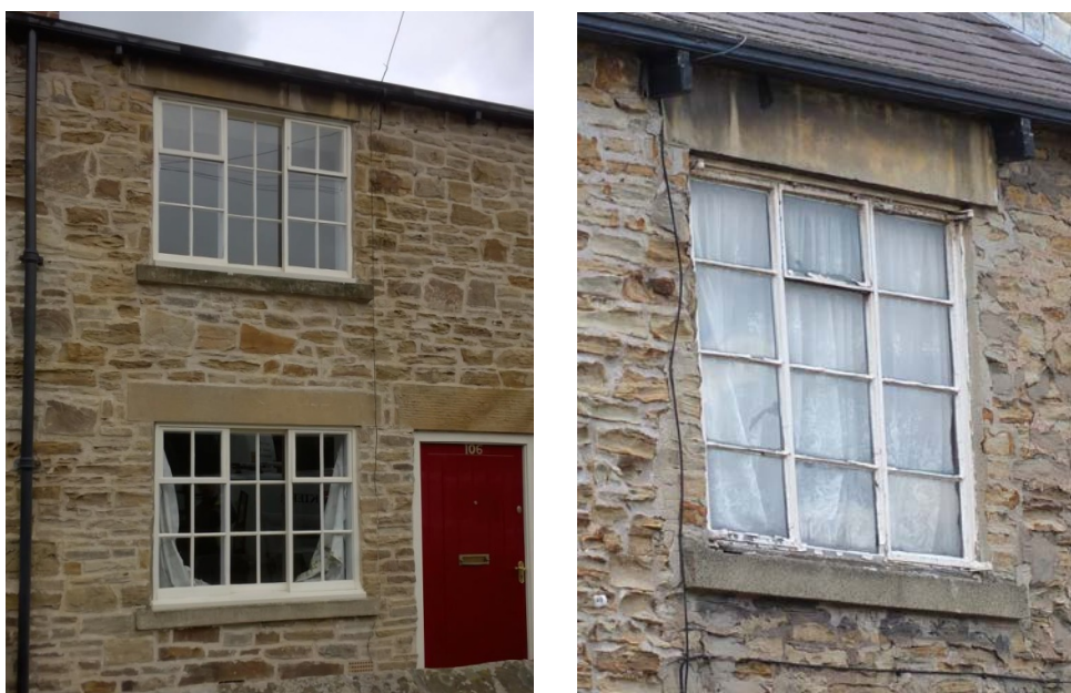
Photos 26 and 27 – Yorkshire sash replacement windows (Reform Row) and metal casement (Station Row)
