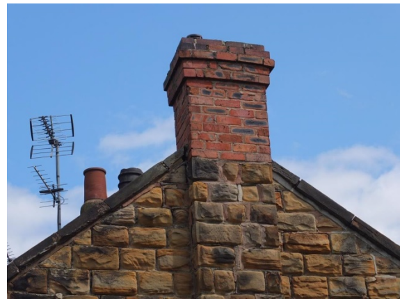
Photo 2 – replaced brick flue with over-sailing courses
