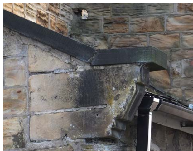
Photo 8 – Kneeling stone at the edge of the gable, supporting the verge coping
