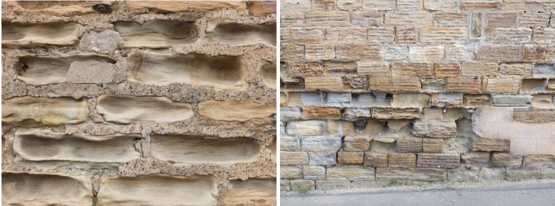
Photos 19 and 20 – damage to stonework caused by use of cement mortar and weathering
