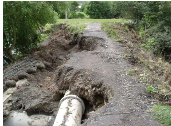
The resulting damage to the dam wall
