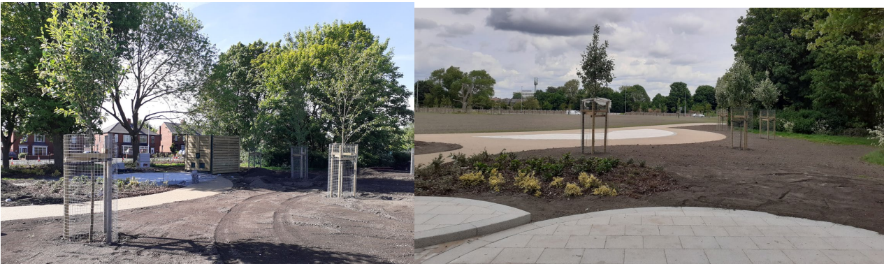
Above: newly cladded cabin and right: patio area for a few chairs and tables for community use
