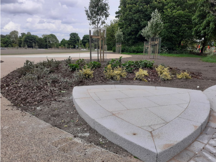
Above: Flexipave footpath towards the park's main entrance, planted area and plinth in front of the newly clad community cabin.
