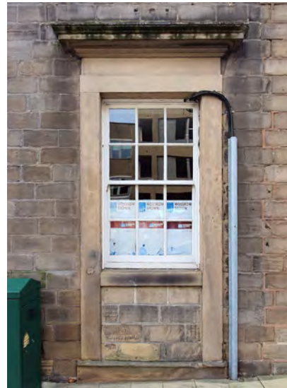
Altered door and intrusive cable trunking
